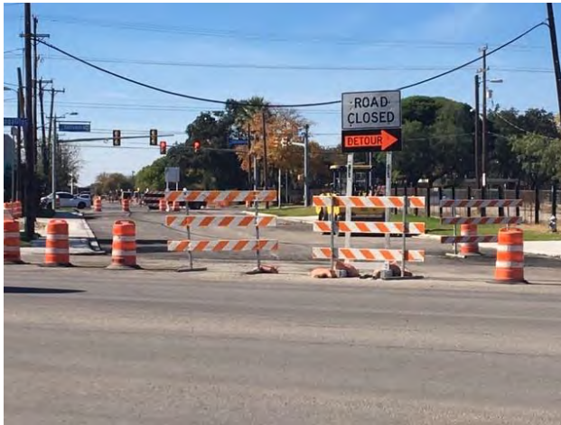
J. Street and sidewalk improvements at Centennial Blvd. between Nogalitos & S. Zarzamora St.
