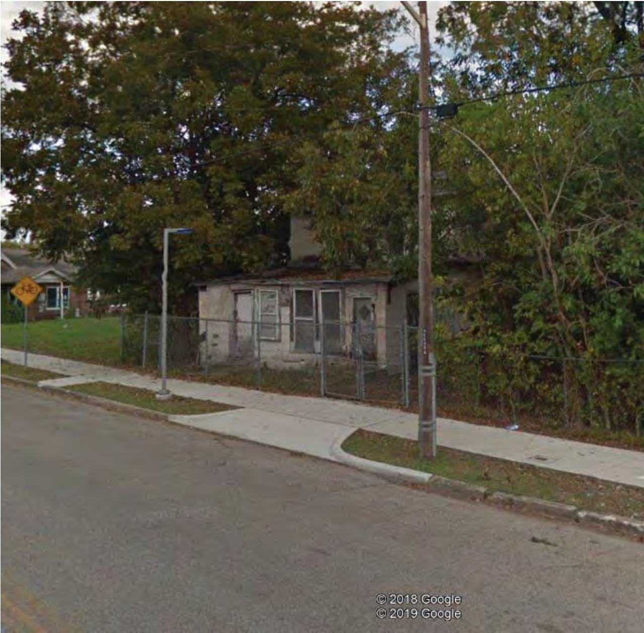
Location B - Home in a state of disrepair within a 1,000-foot radius of our proposed development site.
