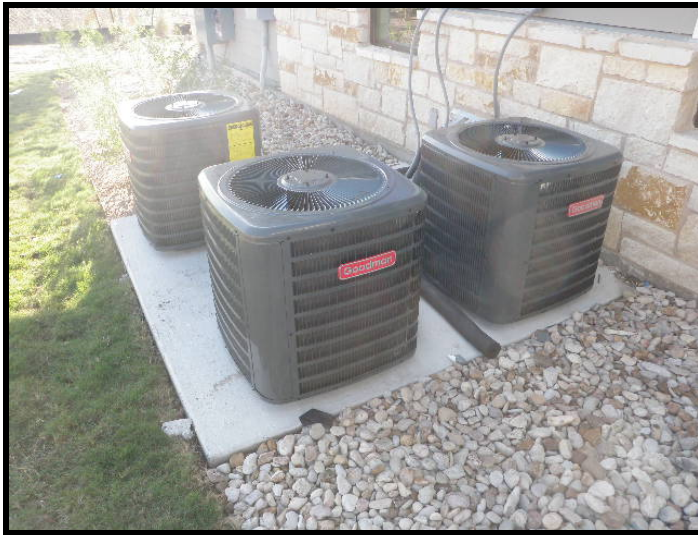
13. Grade mounted condensing units have been installed at Building 6.
