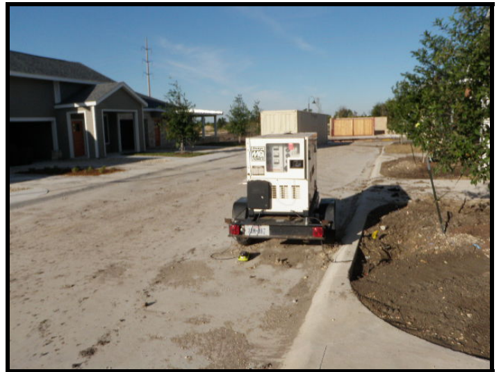
8. Generators remain located on site.
