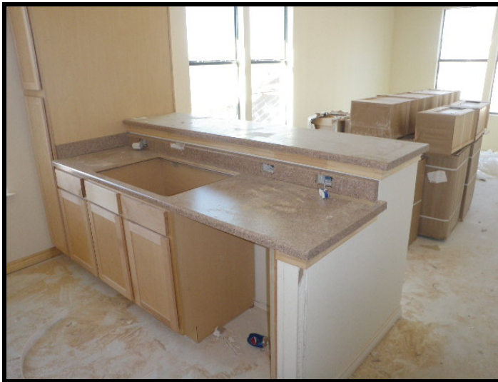
15. Installation of cabinets and countertops was in progress at east portion of Building 1A/B.
