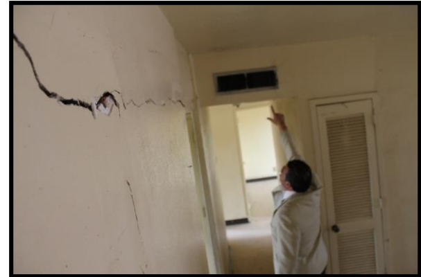
Tays: 11 out of 359 units (3%) offline due to structural damage & asbestos.
