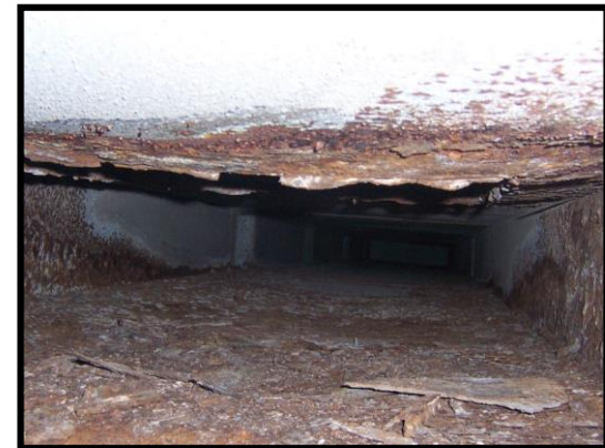
Eisenhower: Rotting ductwork behind asbestos walls and ceilings
