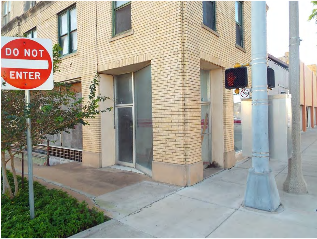
Corner detail of building & sidewalk condition – north east corner.
